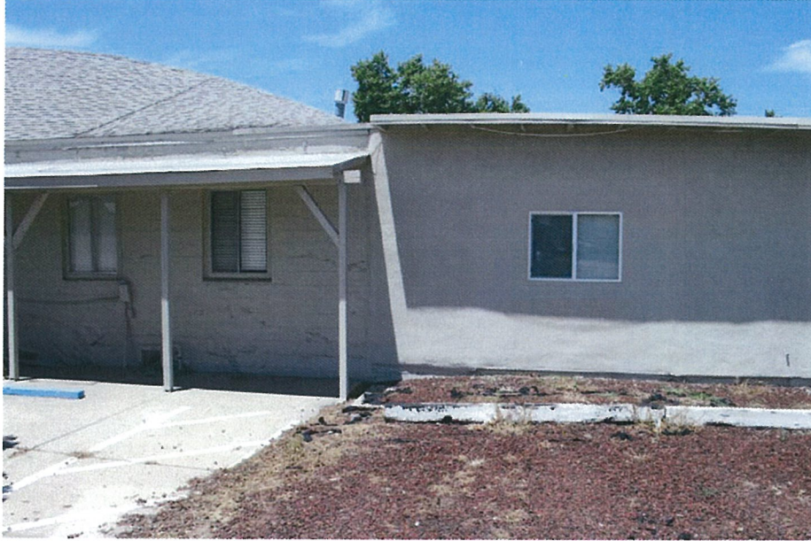
Figure 9: Right rear of the building showing the demarcation where the original 1930 board-formed concrete Hall was extended north with a stucco-clad wood-frame addition.
