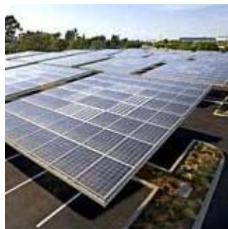
Example of Solar Panel Carport
